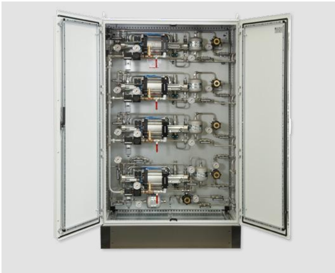
4-stage gas booster station in cabinet design with high pressure gas storage and regulation
